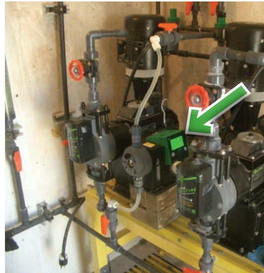
SMART Digital DDA installed at BJWSA, dosing sodium hypochlorite
